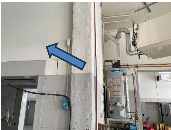
Asbestos-containing asbestos cement (Transite) wall boards (Location 11)
