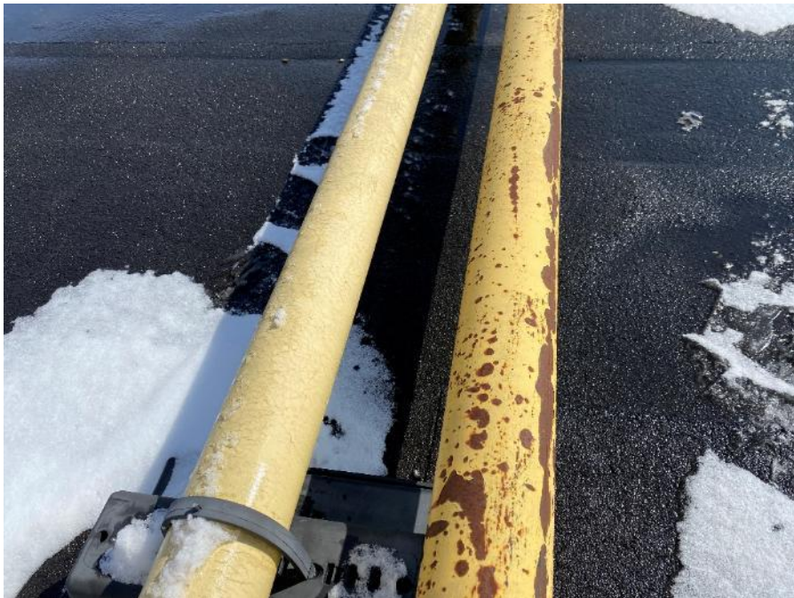
Photo 4 - Yellow paint on metal piping (low lead) and Dark Yellow paint on metal piping (elevated lead)
