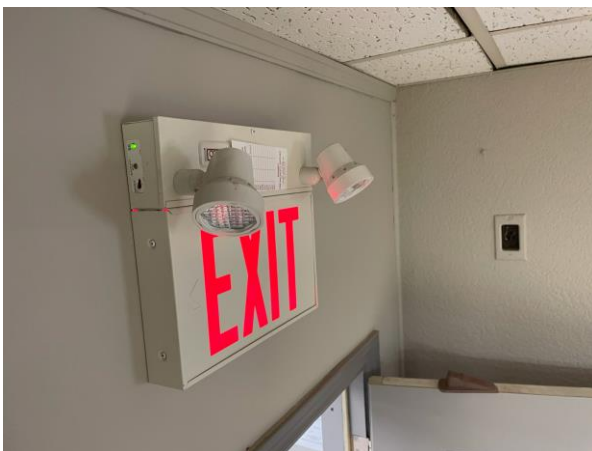
Lead-acid batteries in emergency lighting units
