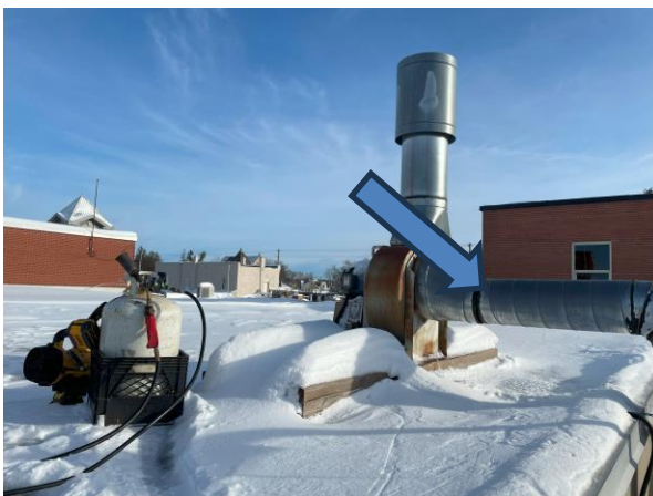
Presumed asbestos-containing black mastic on rooftop ducting
