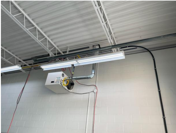
Uninsulated suspended heating units
