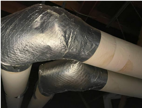
Non-asbestos fibreglass insulations on pipe straights and fittings
