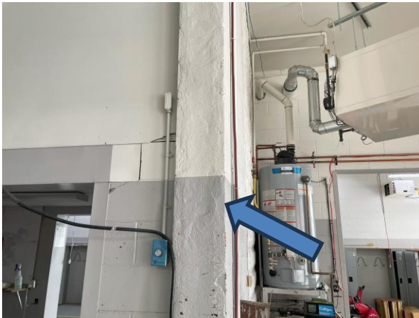
Asbestos-containing texture finish on masonry block wall
